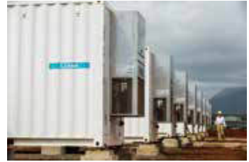
▶ Containerized testing system for BESS Energy group, France
