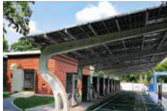
▶ Solar, Storage, Charging and Testing Integrated Solution Municipal investment Group, Guangdong, China
