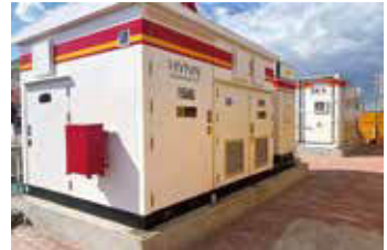
▶ BESS Energy group, Heilongjiang, China
