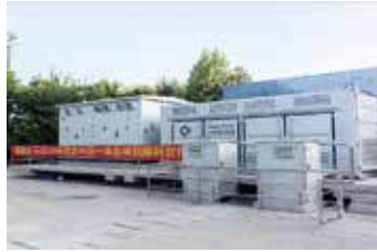
▶ Energy-saving testing for PV station Energy group, Jiangsu, China
