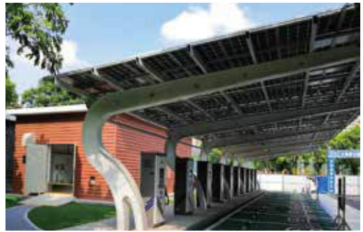
▶ Solar, Storage, Charging and Testing Integrated Solution Municipal investment Group, Guangdong, China
