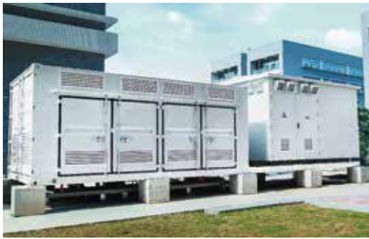
▶ Inverter + step-up boost system Energy group, Jiangsu, China
