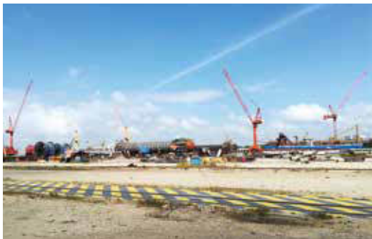
▶ Temporary Power Supply Solution for Construction Site (Middle East Region)
