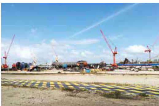
▶ Temporary Power Supply Solution for Construction Site (Middle East Region)
