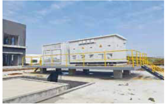
▶ Inverter + step-up boost system Energy group, Inner Mongolia, China
